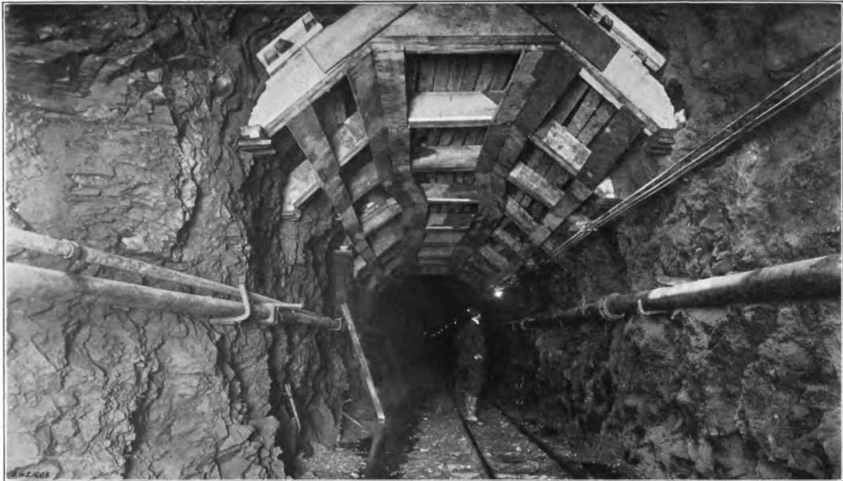
SHANDAKEN TUNNEL.—Temporary timbering in the north tunnel at Shaft 3. The heading at this point was excavated through mixed red and gray shaly sandstone. The timber was placed three months after the excavation had been done.
