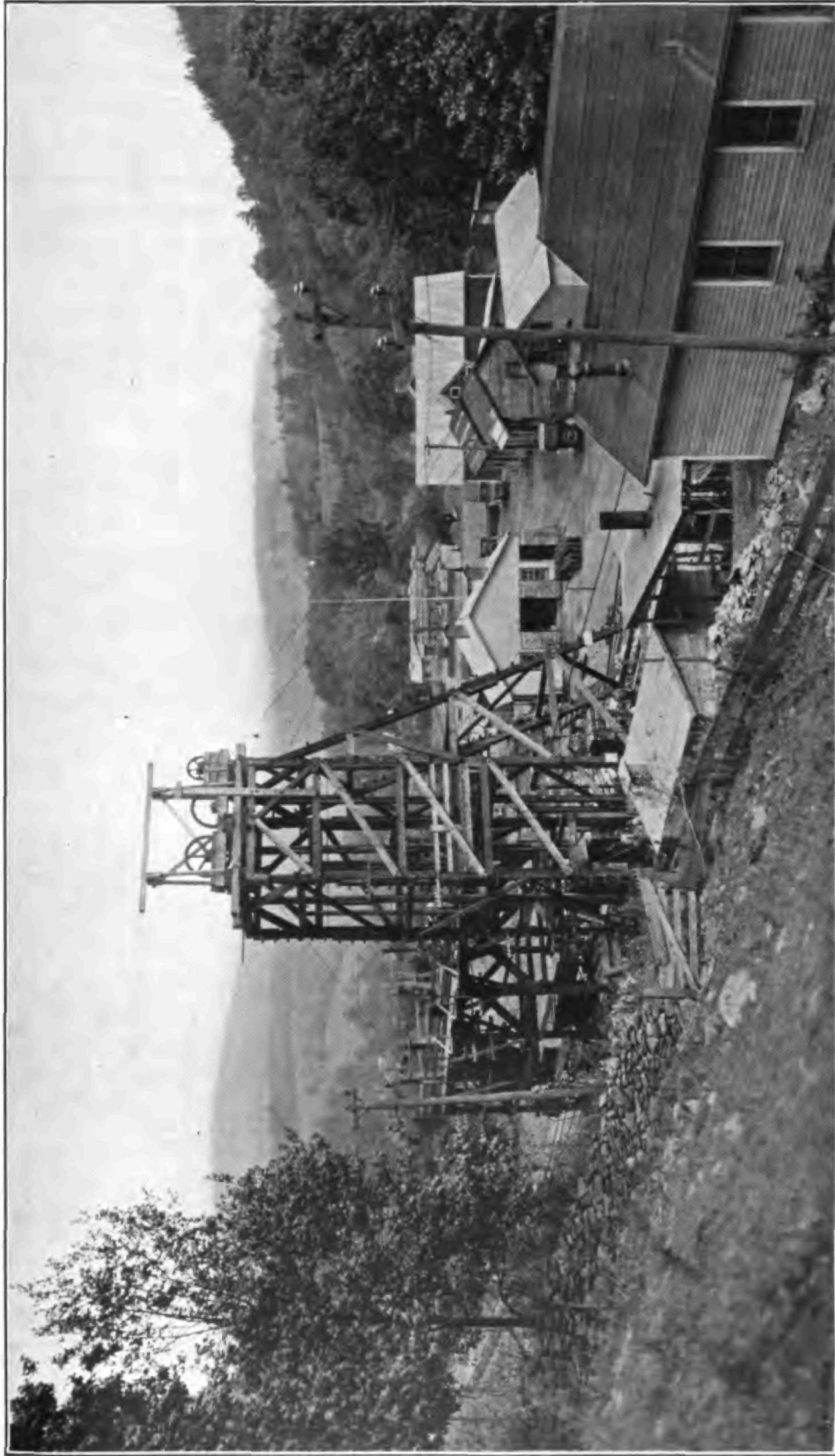
SHANDAKEN, TUNNEL.—General view at Shaft 4, showing the head-frame, plant and buildings at top of the shaft.
