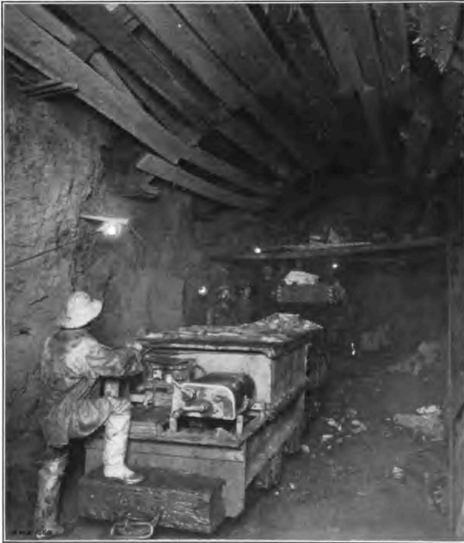
SHANDAKEN TUNNEL—South tunnel at Shaft 6. The tunnel muck is removed by the mucking machine which loads it into the cars which are in turn hauled to the shaft by the storage-battery locomotive. The platform in background is for use in placing permanent timbering.
