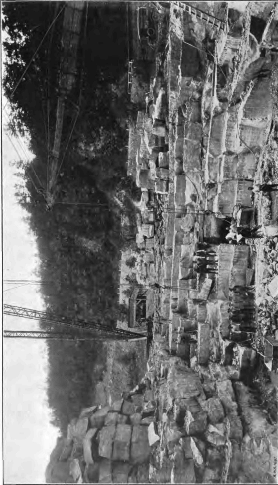
SCHOHARIE RESERVOIR.—The Riverside quarry, where stone is obtained for the construction of the Gilboa dam. The stones shown have been quarried and are ready to be dressed.
