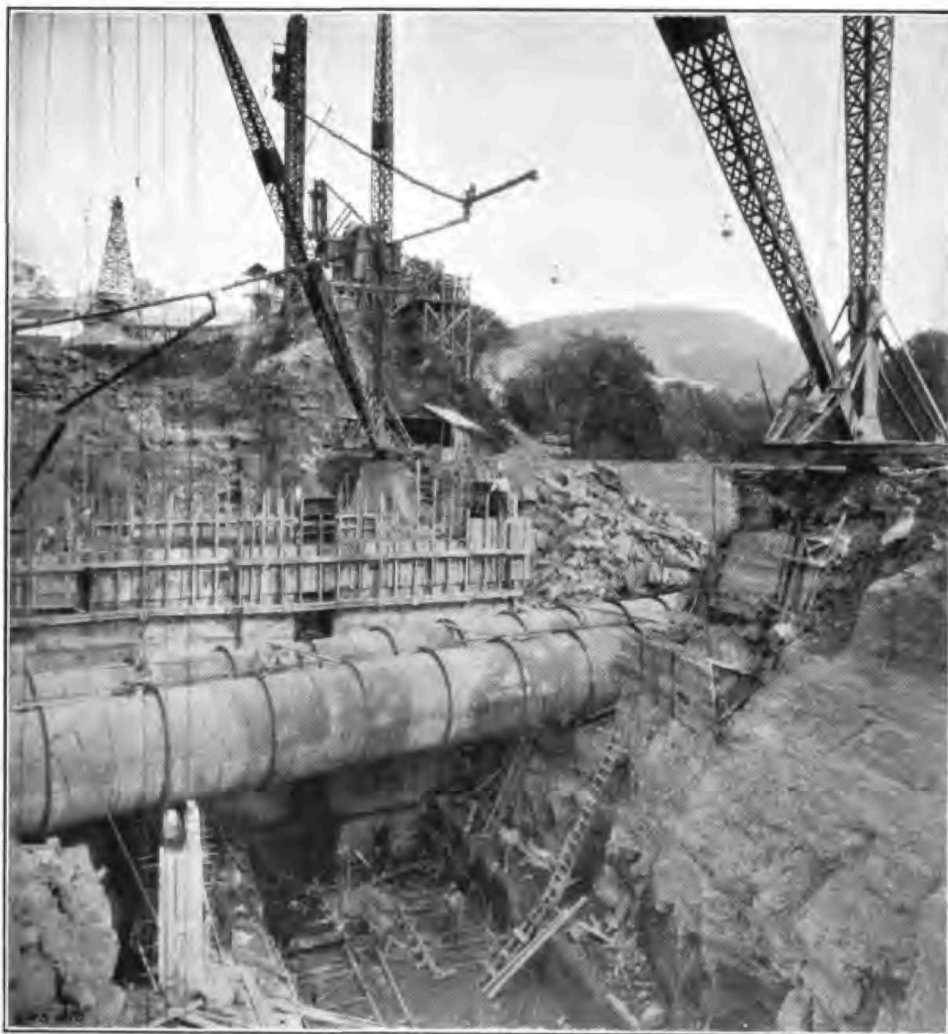
SCHOHARIE RESERVOIR—Excavation for the Gilboa dam, looking easterly, showing the cut-off trench below the 9-foot stream-control pipes which temporarily carried the flow of the Schoharie creek. Beyond the pipes work is in progress on placing concrete masonry in the dam.
